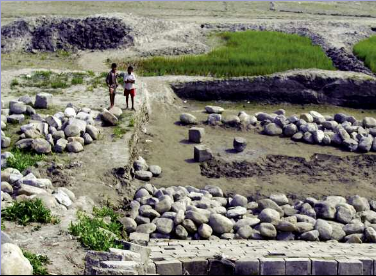
River bank protection activities along the Brahmaputra River, Bangladesh, that completely dries up during the dry season and floods over during the rainy season.
